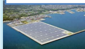
Solar power station
