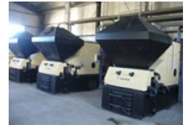
High-efficiency Heat only Boilers, Suuri-Keikaku, Mongolia
