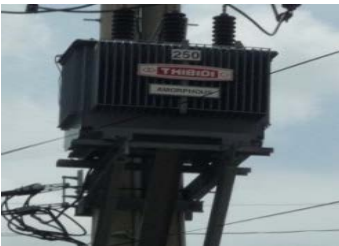
Amorphous transformers in power distribution, Hitachi Materials, Viet Nam
