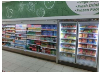
Energy saving at convenience stores, Panasonic, Indonesia
