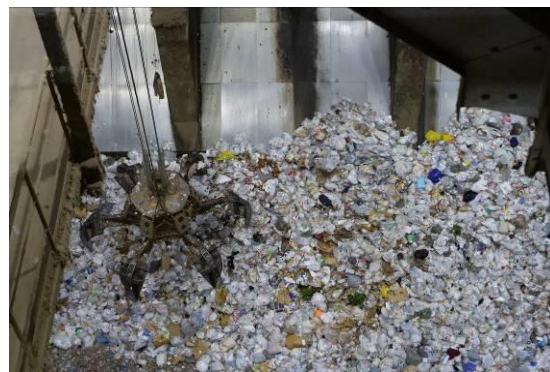
Photo 4-37 (2) Inside the Waste Pit
