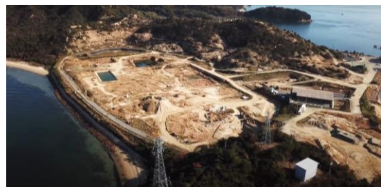
Photo 5-4 Bird's Eye View of the Illegal Dumping Site (November 2021)
