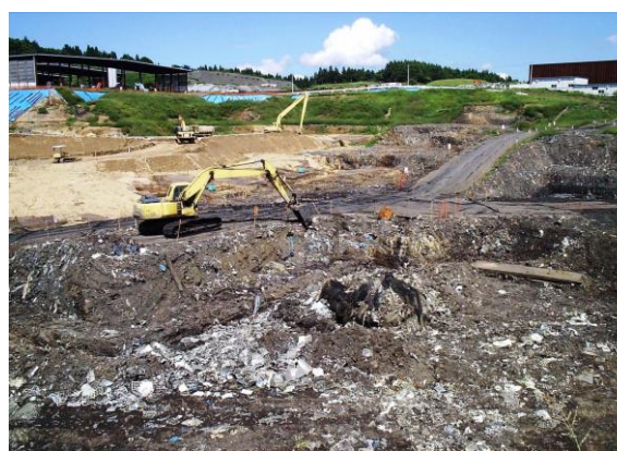
Photo 5-8 Situation of Illegal Dumping (2012)
