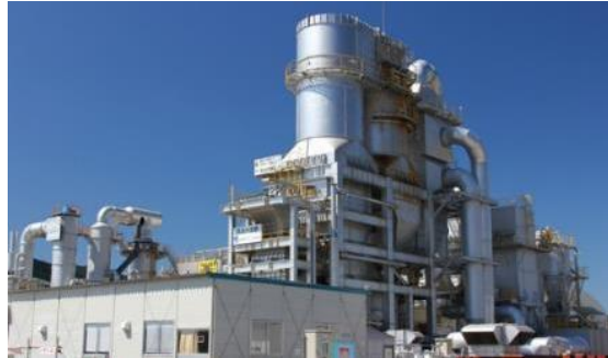
Photo 5-12 Temporary Incinerator (Koizumi Region, May 2013)
