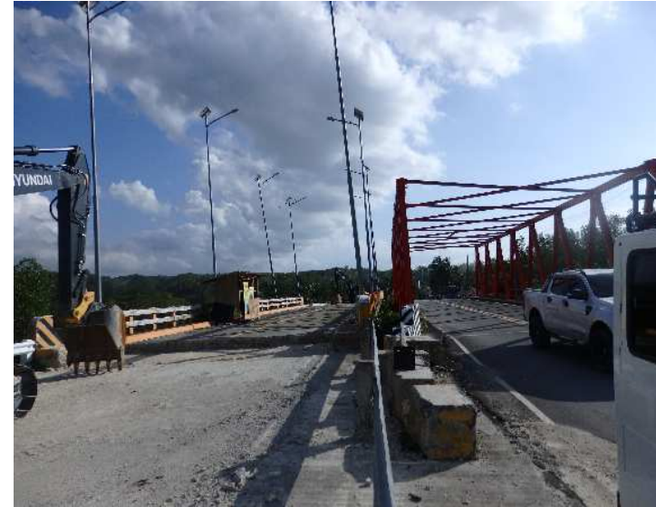
Photo6. Settlement at the abutment②
