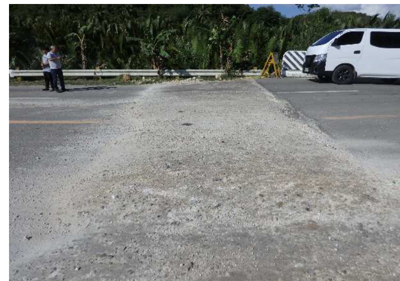
Photo4. Settlement at the abutment②
