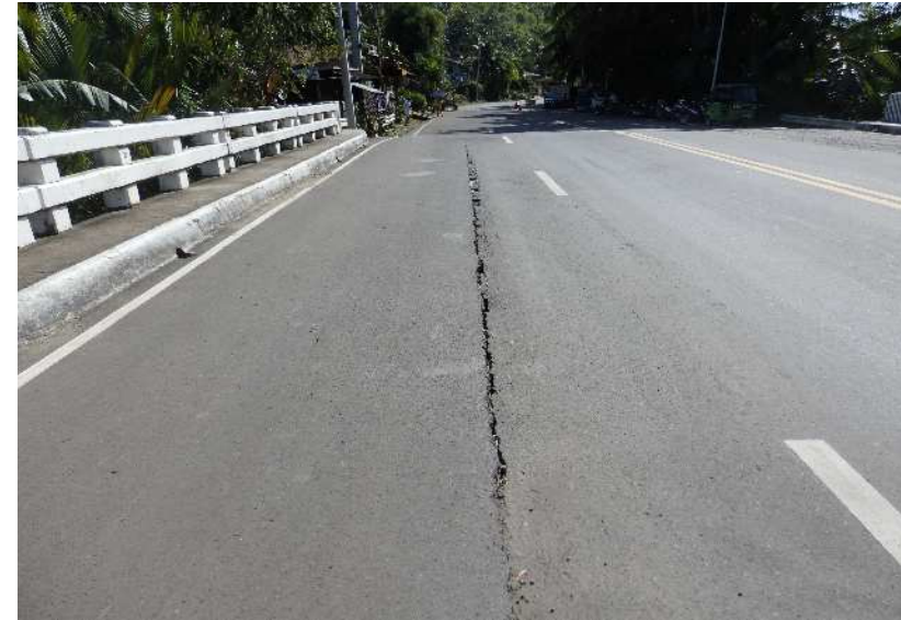
Photo2. Crack at longitudinal joint between deck slab of inner bridge and widening bridge②
