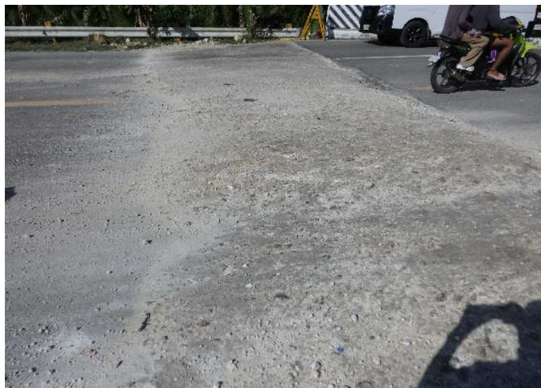
Photo3. Settlement at the abutment①
