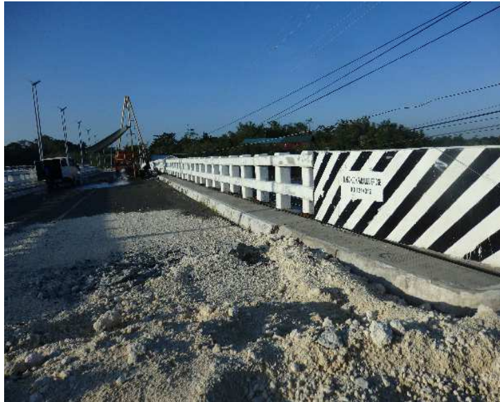
Photo9. Settlement at the abutment
