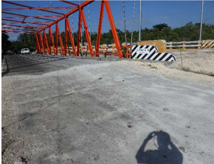
Photo5. Settlement at the abutment①
