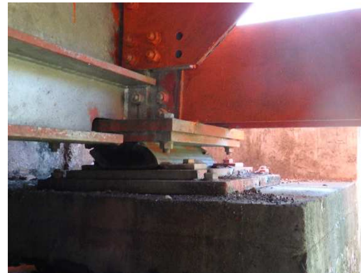
Photo8. Damage to the bearing
