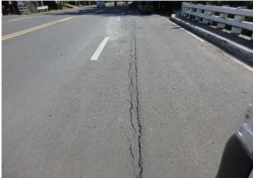
Photo1. Crack at longitudinal joint between deck slab of inner bridge and widening bridge①
