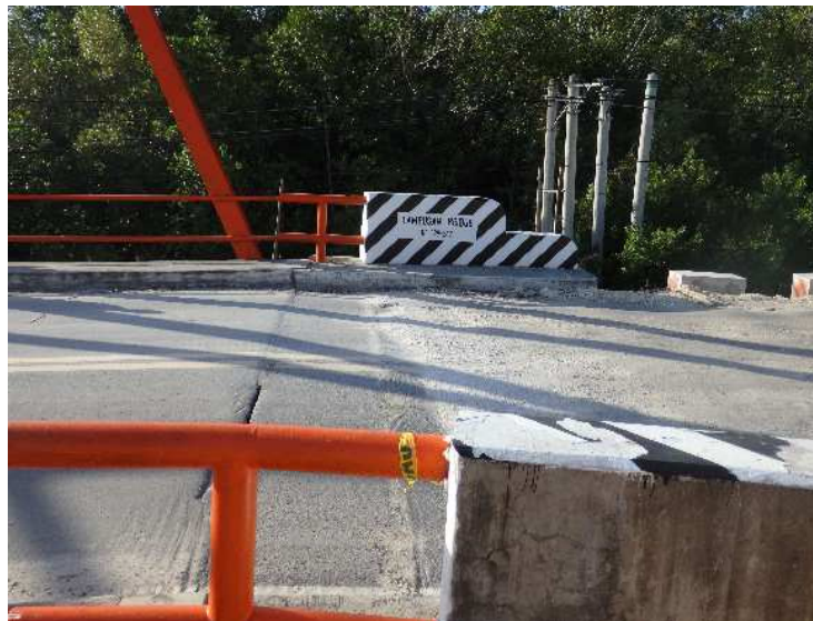
Photo7. Settlement at the abutment
