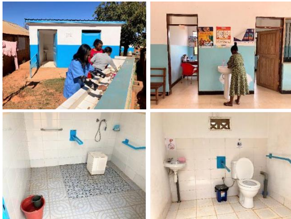
Figure 9: Examples of improved WASH facilities in health care facilities
