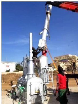
Senegal Installation of medical incinerator
