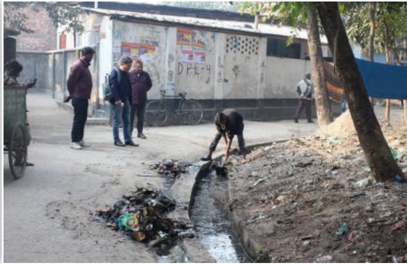
Action Plan monitoring activities on Drainage cleaning at ward no.24 at GCC
