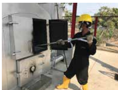
Operation of Incinerator (16, January 2022)
