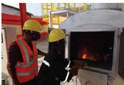
Operation of Incinerator (11, January 2022)
