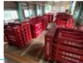
Hydrogen (accumulation container)
