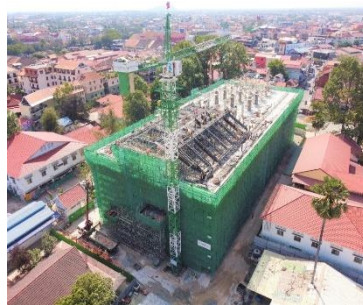
A general view from northwest side of the construction facility at the Siem Reap Provincial Hospital.
