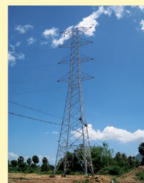
Power Transmission and Distribution Tower
