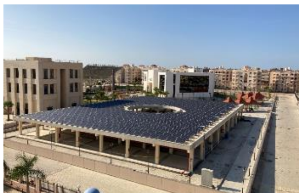
Solar PV Station
