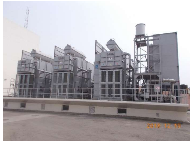
In Ghana, JICA is supporting to upgrade a substation for stable power supply.
