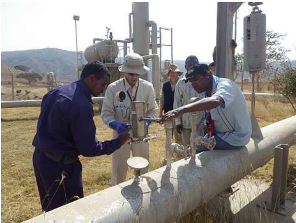
JICA is supporting capacity building for geothermal development in Ethiopia, a country with abundant geothermal resources. The photo shows steam extraction at the Aluto Langano geothermal power plant.
