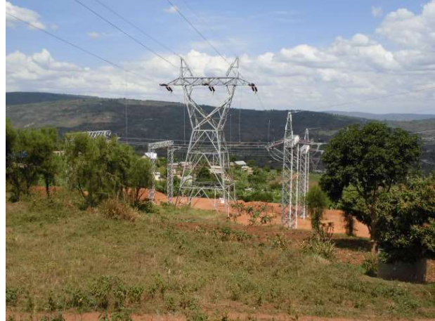
JICA is supporting the renovation and expansion of the power transmission and distribution network to stabilize and improve the efficiency of the power supply in Rwanda.
