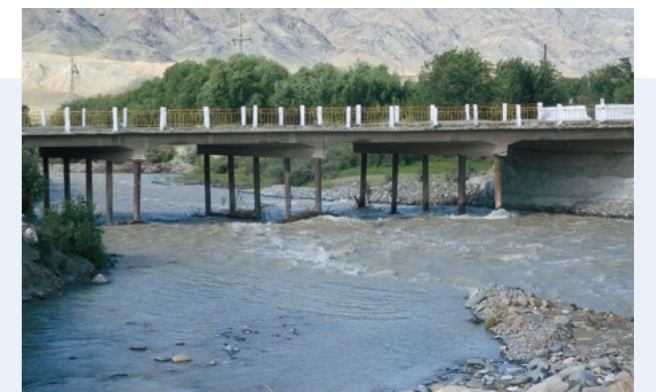
The deteriorating Urmalar River Bridge, prior to reconstruction
