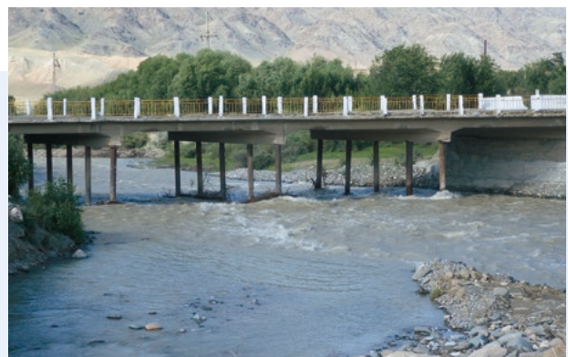
The deteriorating Urmamal River Bridge, prior to reconstruction
