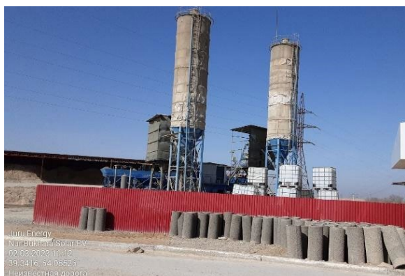
Figure 46: Photo of batch plant
