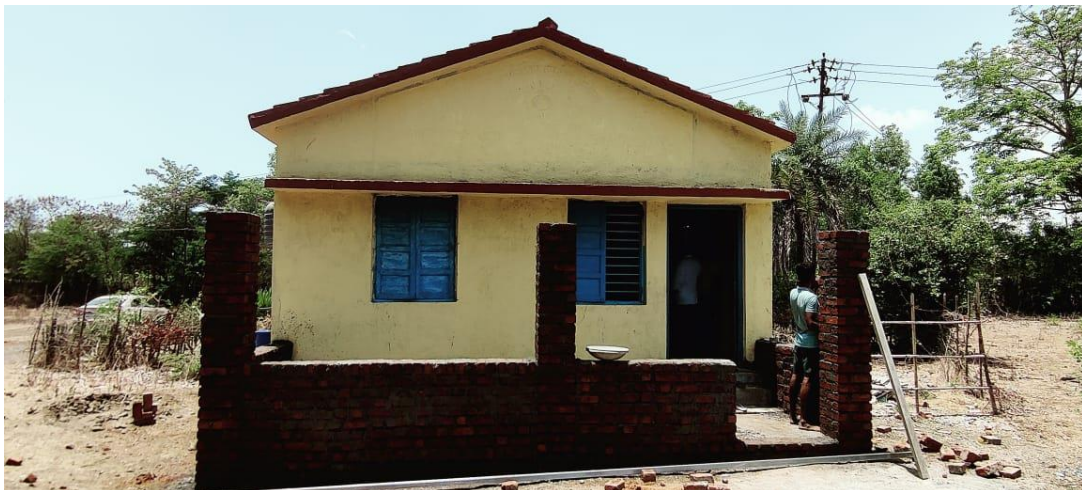
Date: 8 th June 2023, Site visited at Machipada Vanai village, Dahanu Tehsil, District Palghar "Village Development Program" under verified Anganwadi repairing work nearby completion.
