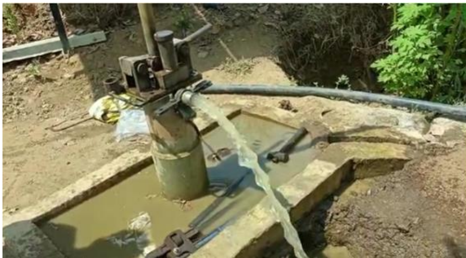
Date: 26 th May 2023, Site visited at Nagale village, Vasai tehsil, Palghar district “Village Development Program” regarding drinking water facility solar energy work is in under progress
