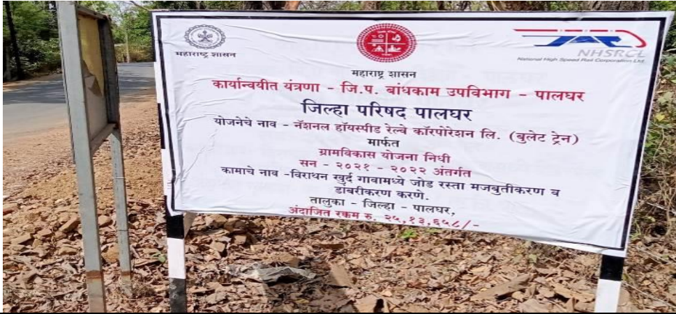
Date: 22 nd June 2023, Site visited at Viratan Khurd, Tehsil District Palghar "Village Development Program" under asphalt road construction work completed.
