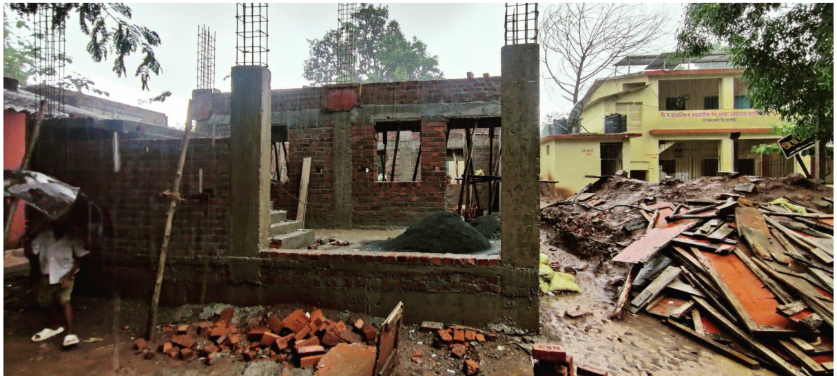
Date: 28 nd June 2023, Site visited at Patilpada Amgaon village Tehsil Talasari, District Palghar "Village Development Program" under Zilla Parishad School classroom construction is in progress.
