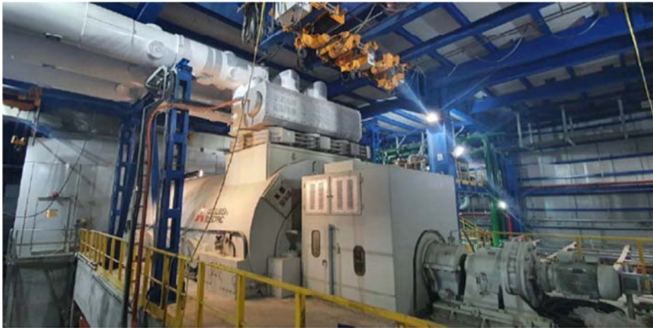
Turbine a Gaz
