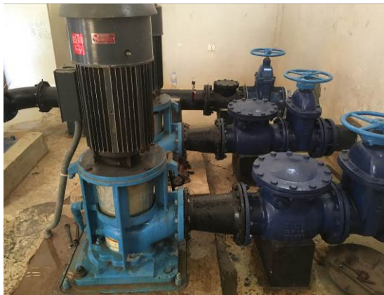
Photo1-3 : Existing Intake Pump (June 2017)
