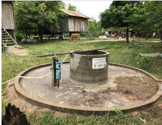
Photo4-1 : Shallow well drilled in each commune. People has not use it because of drying up (July 2017)
