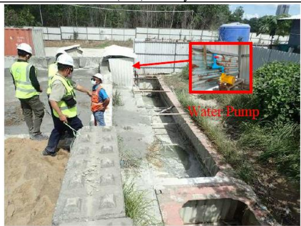
Photo 4: Provisional Tank for Contaminated Water at Chip Mong Concrete Mixing Plant in May 2024
