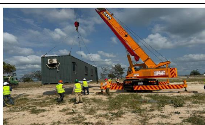
Photo 2: Mobilization of equipment for Temporary's Facilities in the Temporary Yard in April 2024
