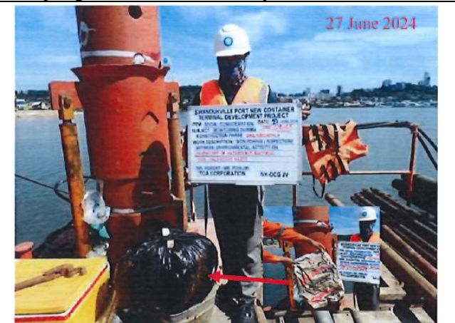
Photo 12: Bentonite Bag in Sealed Black Plastic in June 2024
