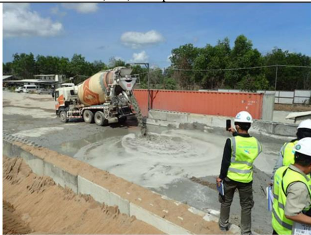
Photo 3: Mixer Truck Cleaning of Ball Drum and Chute at Chip Mong Concrete Mixing Plant in May 2024
