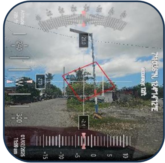
SOLAR LIGHT PANEL (4)
