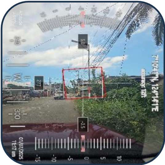
SOLAR LIGHT PANEL (8)
