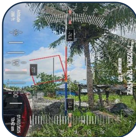
SOLAR LIGHT PANEL (3)
