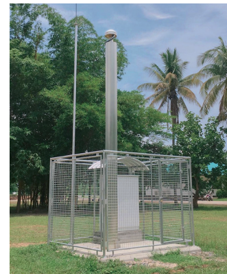
A satellite-based continuous observation reference station in Thailand. It houses antennas, receivers, and communications equipment that receive satellite signals.
