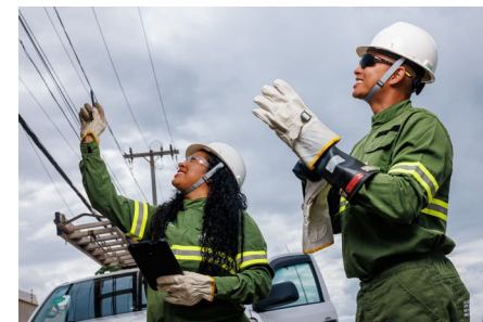
Female electrical engineer inspecting distribution network
