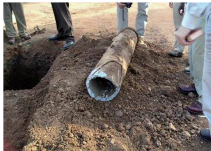
Broken water line. Photograph courtesy of JICA
