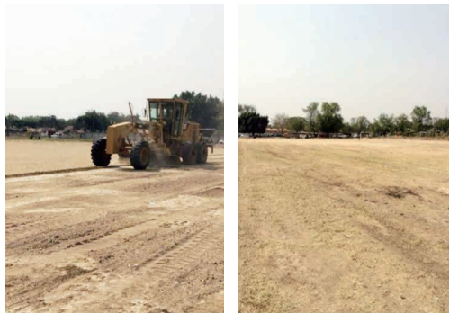
Construction equipment of CTI Engineering International Company, which is doing grant aid work in South Sudan, being used to prepare grounds in Juba City with the assistance of the Central Equatoria Ministry of Infrastructure.
