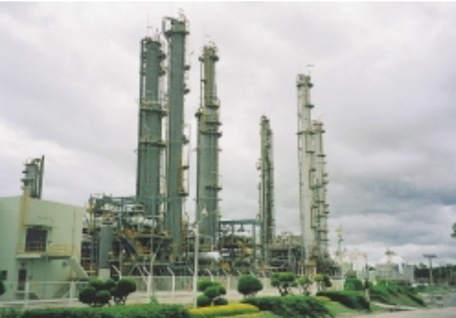
Gas Separation Plant in Map Ta Phut Industrial Complex
