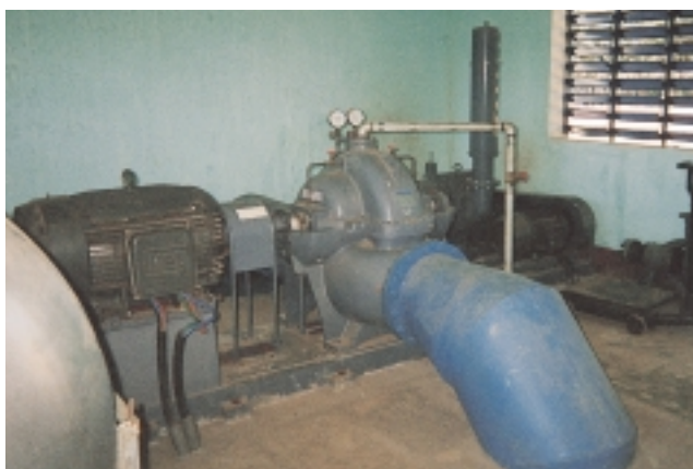
Large Pumps procured by this Loan
