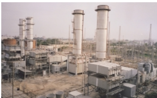
General View of Basin Bridge Power Station
