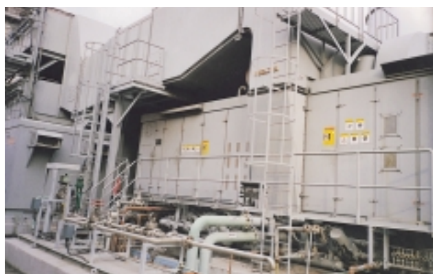
Gas Turbine Generator
