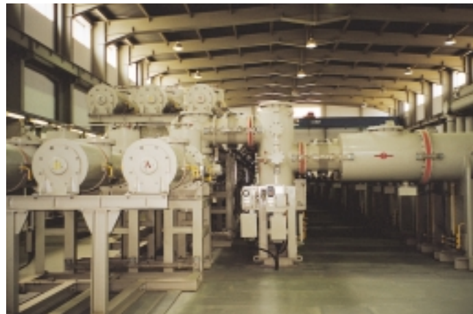
Gas Insulation Switchgear
