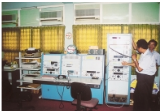
SAR Telecommunication Equipment
