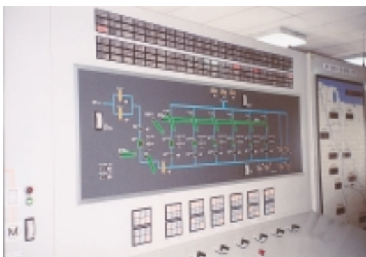
Control Panel Inside the {Sarinah Thamrin} Pumping Station
