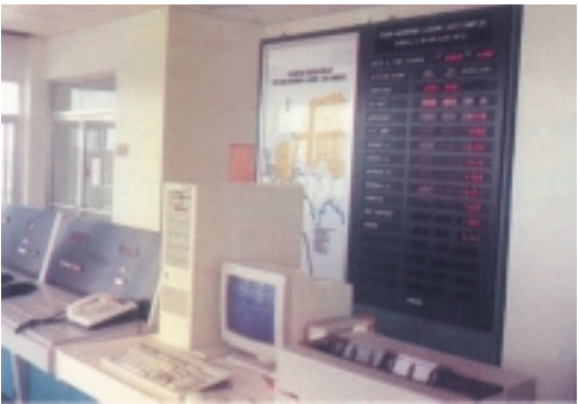
Rosario Central Monitoring Facility
