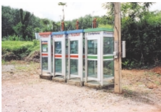
Public Telephone Installed by the Project
