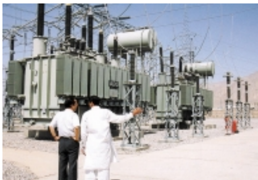
Industrial II Transformer Station
