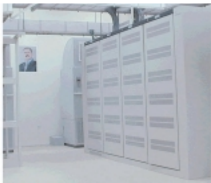
Switchboard Equipment Installed by the Project
