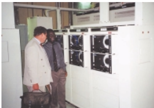
PTC Harare Central Switchboard Station
