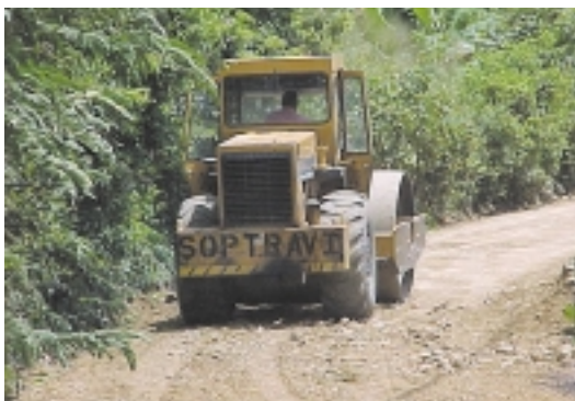
Procured Equipment in Use
