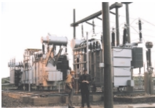
Equipment Installed by the Project
