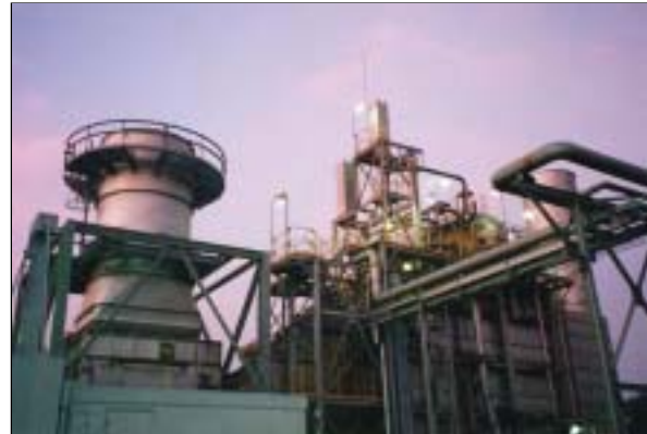
Site Photo: No.2 Gas Turbine
