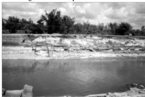
Figure-3: Collapsed Embankment of MMC
