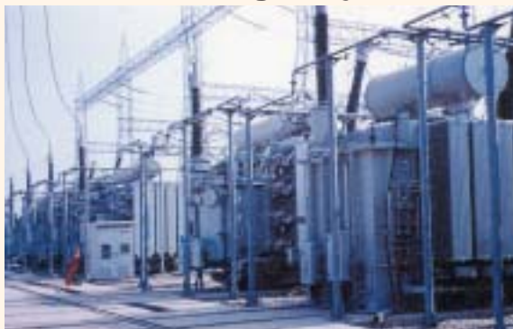
Substation at Multan
