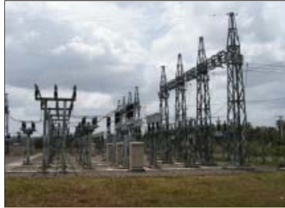
Site Photo: Matara Substation
