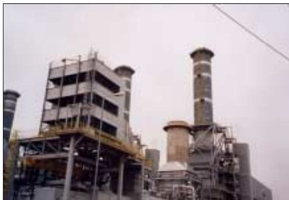
Site Photo : Combined Cycle Power Station
