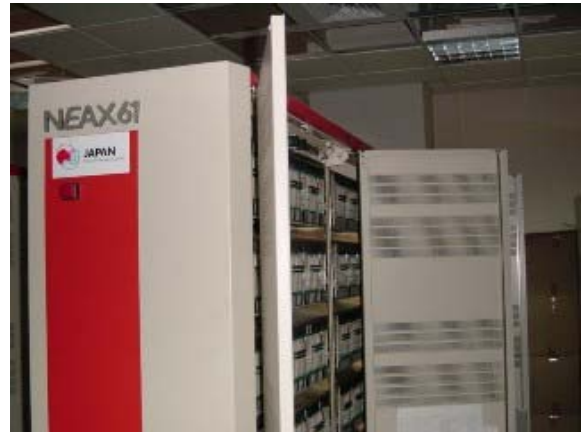
Switchboard System (Accra Station)
