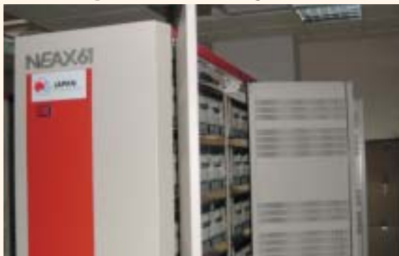
Accra Telephone Exchange Station
