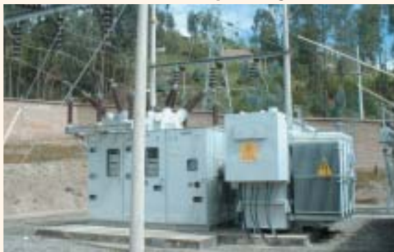
A sub-transmission station
