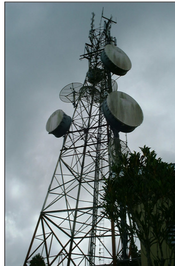
Site Photo: Microwave Transmitter
