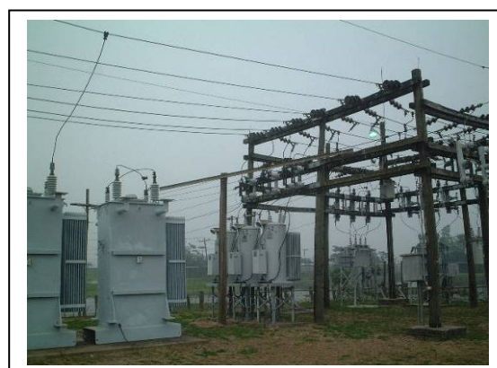
Sunamganj PBS power substation
