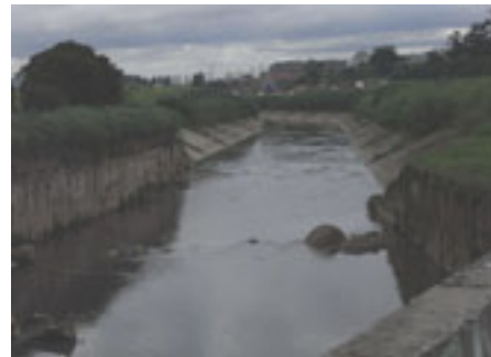
Figure 15: Cross-sections of the Cabuçu de Cima River. The near side is rectangular concrete, and the
