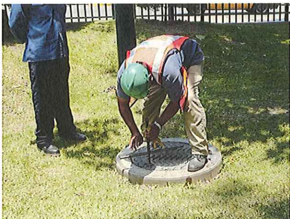
Manhole for the underground water distribution valve chamber at a public park
