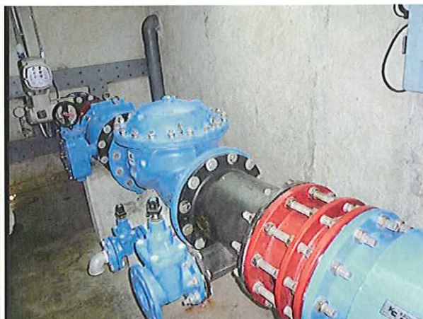
Remotely controlled water distribution valve
