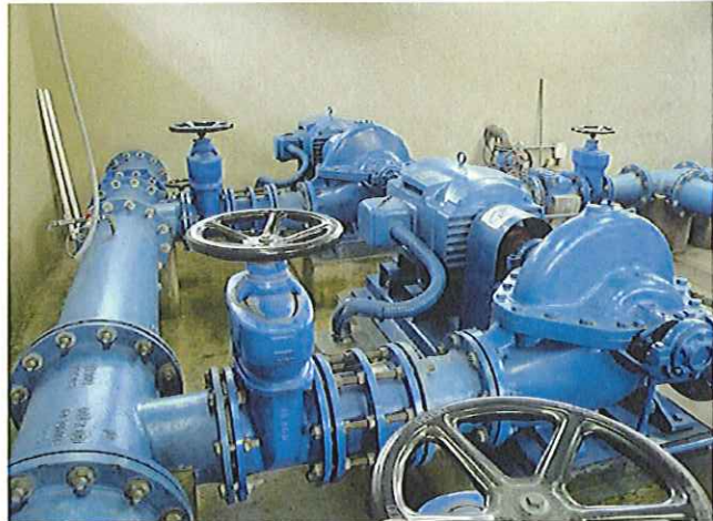
Water distribution pump (Rimac District, Lima)
